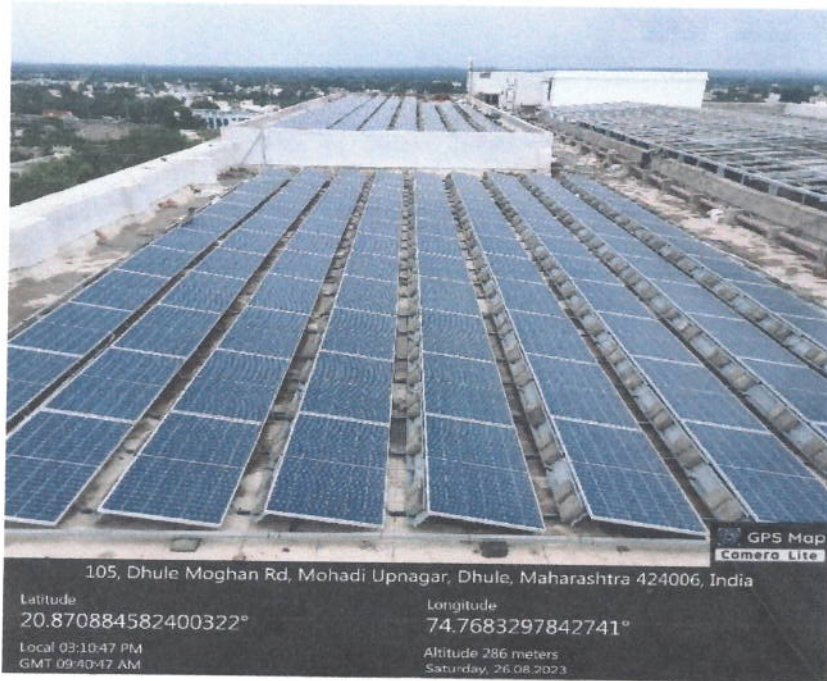
Photo. A view of photovoltaic panels set-up on Institute's Rooftop – 26/08/2023
