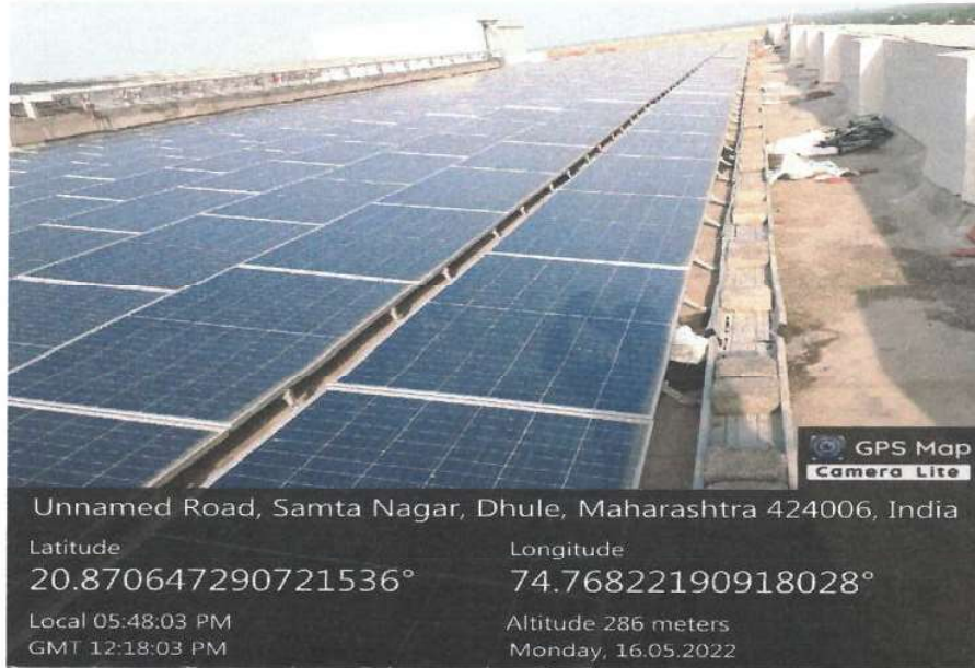
Photo. A view of photovoltaic panels set-up on Institute's Rooftop
